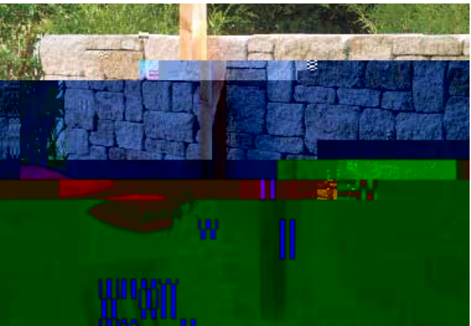
Split masonry bricks
